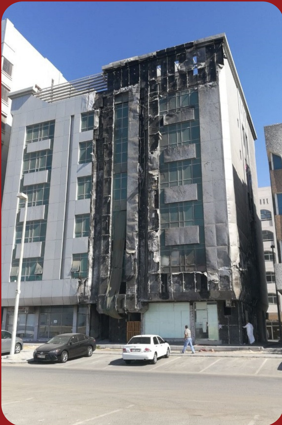
Fired façade of a residential building before repair
